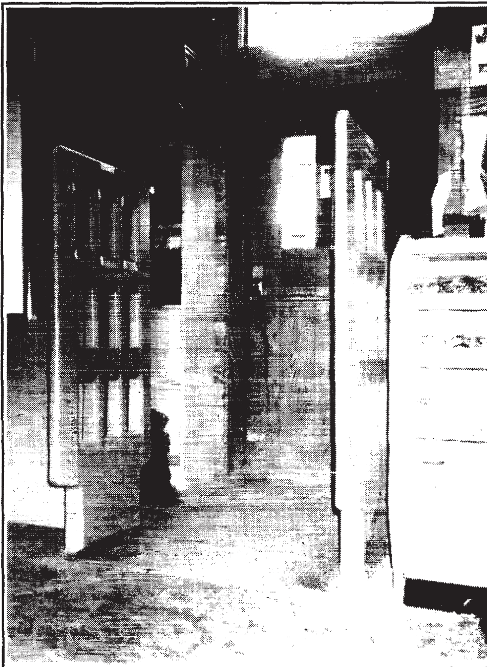
This magnetic "inventory control system" was recently re-installed at the bookstore to curb theft.
