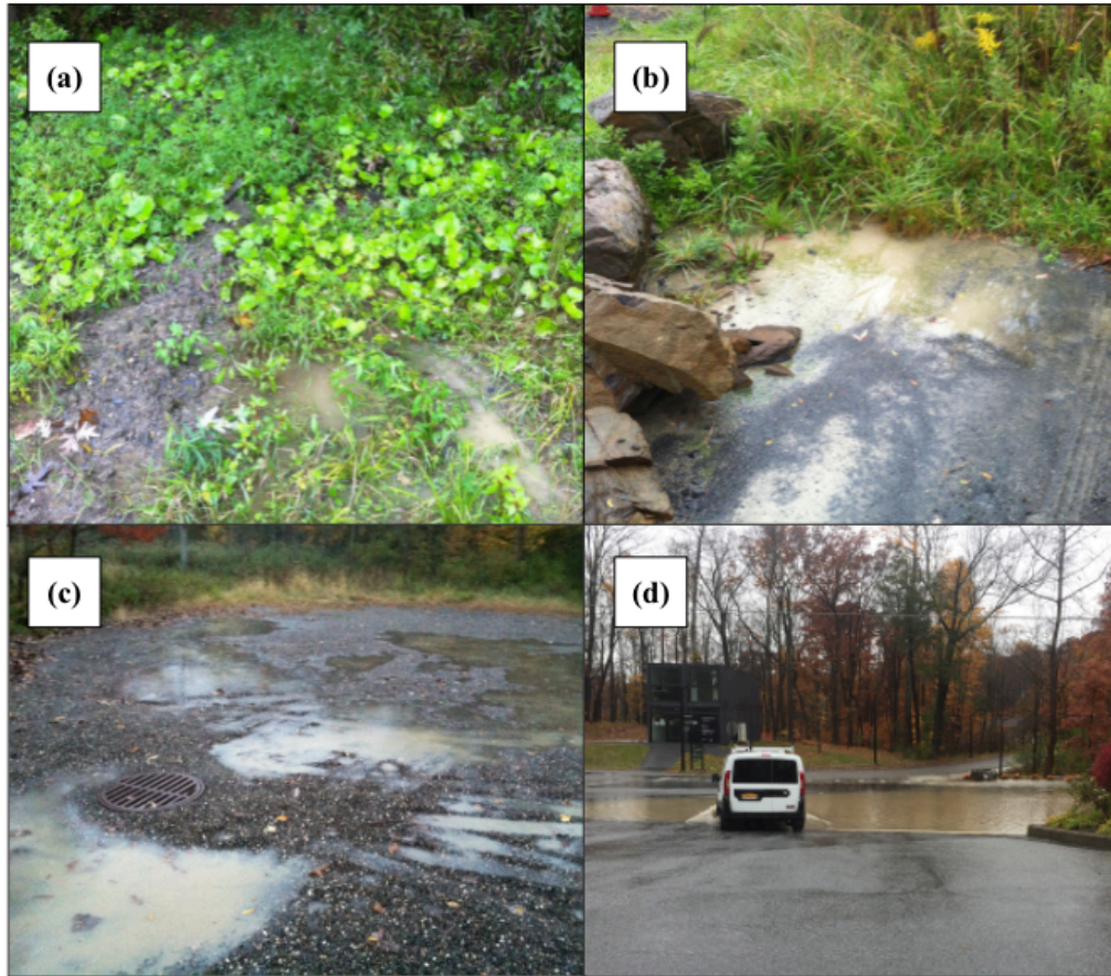
Figure 4.1: (a, b, c) Site of GI project prior to installation showing flooded areas and erosion of the gravel parking area (d) Flooding of another parking area on Bard's campus (Nov. 2018).
