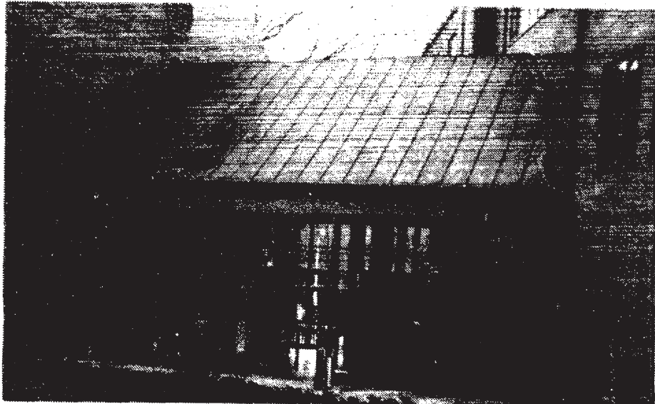
This anteroom leaks when it rains.
