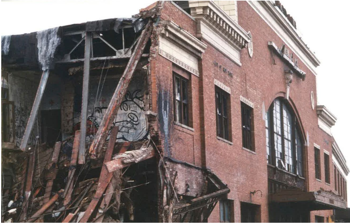
Figure 2.22. Pier 34's demolition in 1984 and you can see Wojnarowicz's mural on the verge of being erased from history. 1984. In Pier 34 . 205 Hudson Gallery, New York, NY
