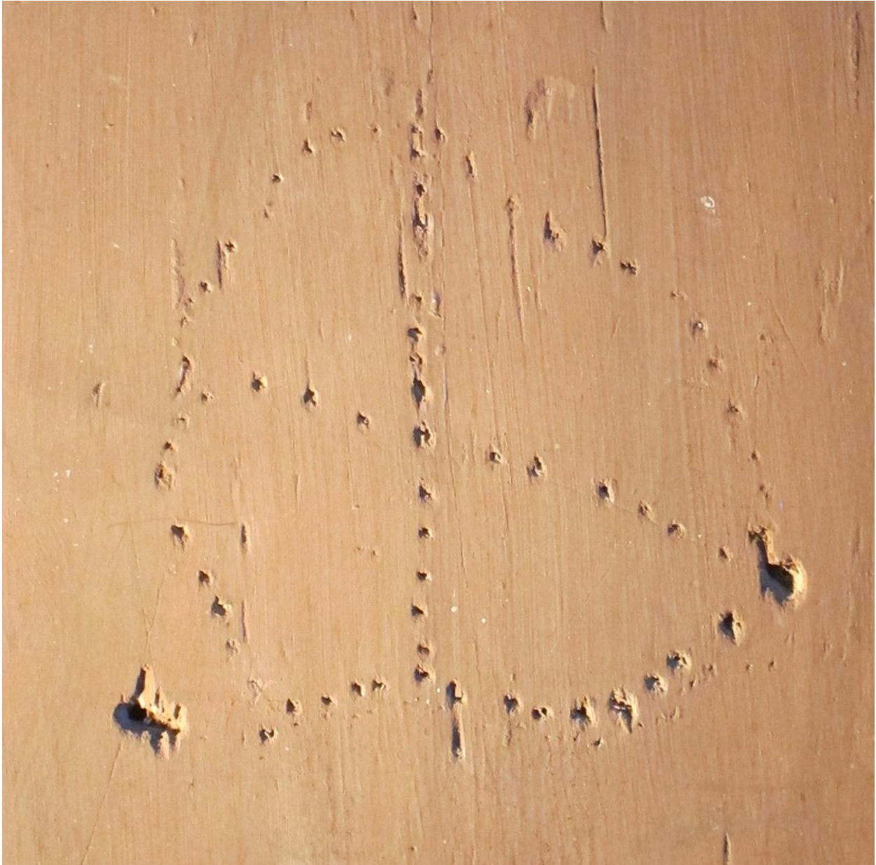
Figure 10: The dikenga located on the right-side vertical frame of the hearth in the Germantown Parsonage.
