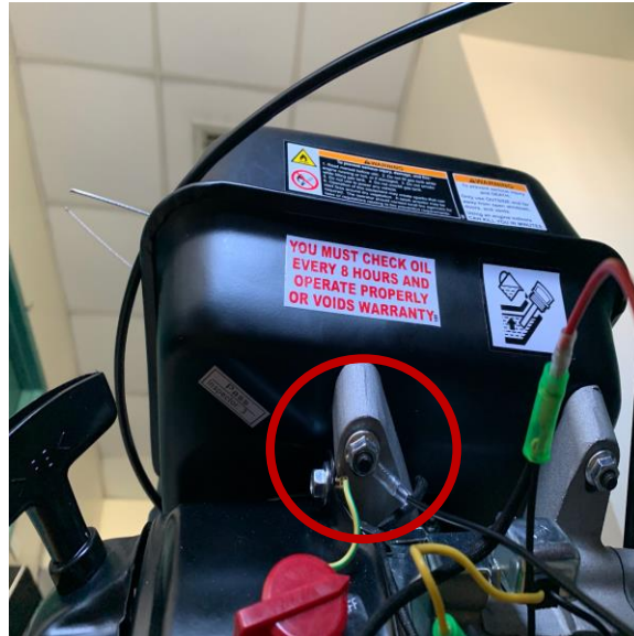
Figure 3.9.2 Grounding the switch
