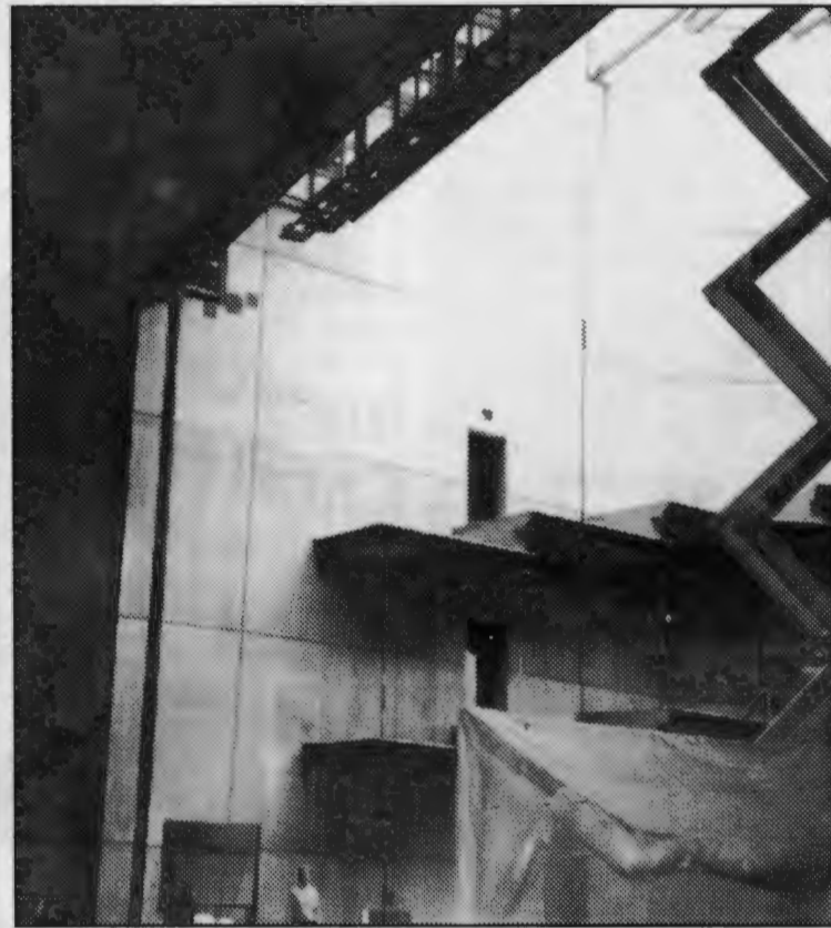
The work of a modest man: A shot of the massive interior of the Gehry Performing Arts Center, nearing completion.
