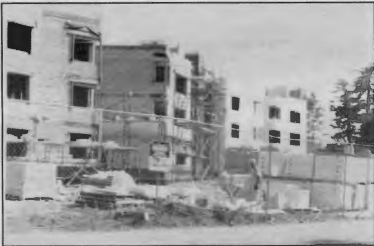
Body storage: The shape of the New Toasters can be made out, but the construction is far from complete.
