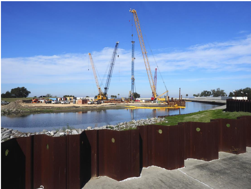
12. Construction of a new lakeshore pumping station at Orleans Ave. Canal, New Orleans.
