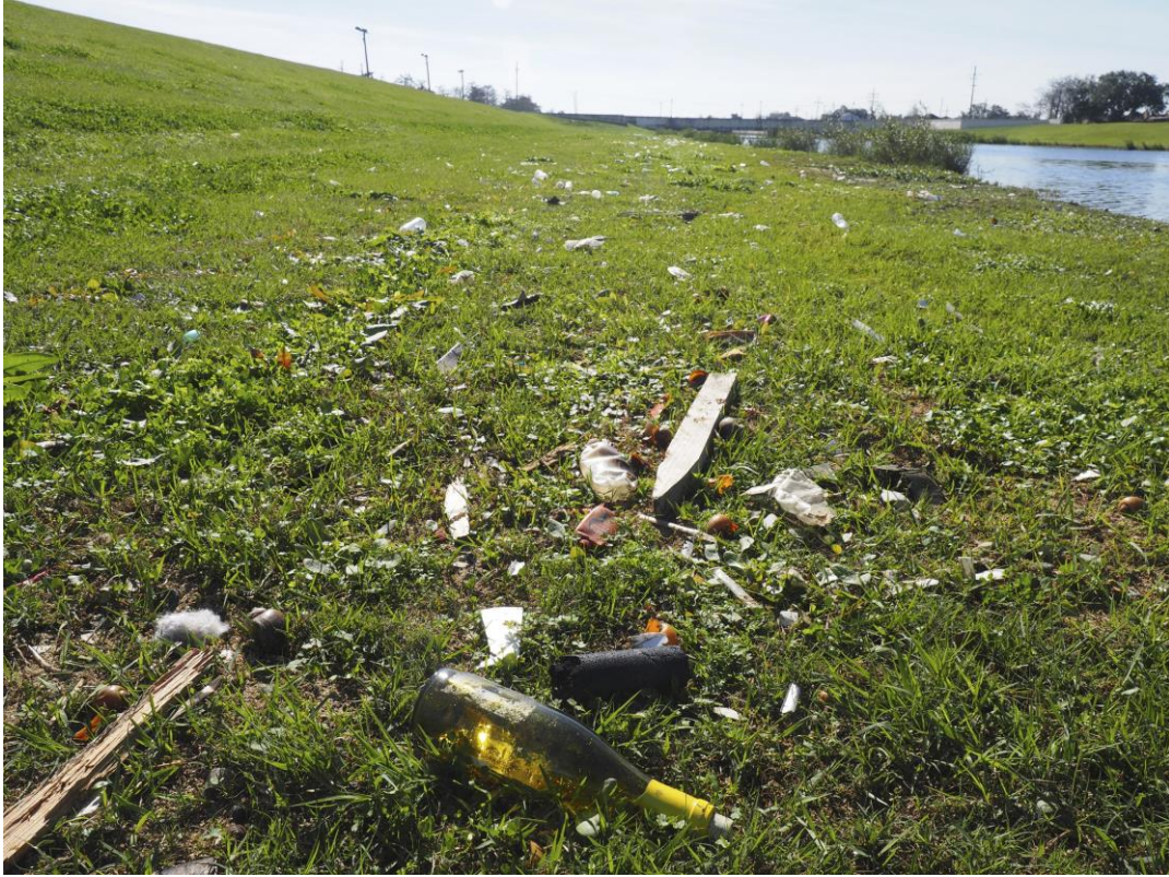
11. Trash along the interior of a guide levee at Orleans Ave. Canal, New Orleans.
